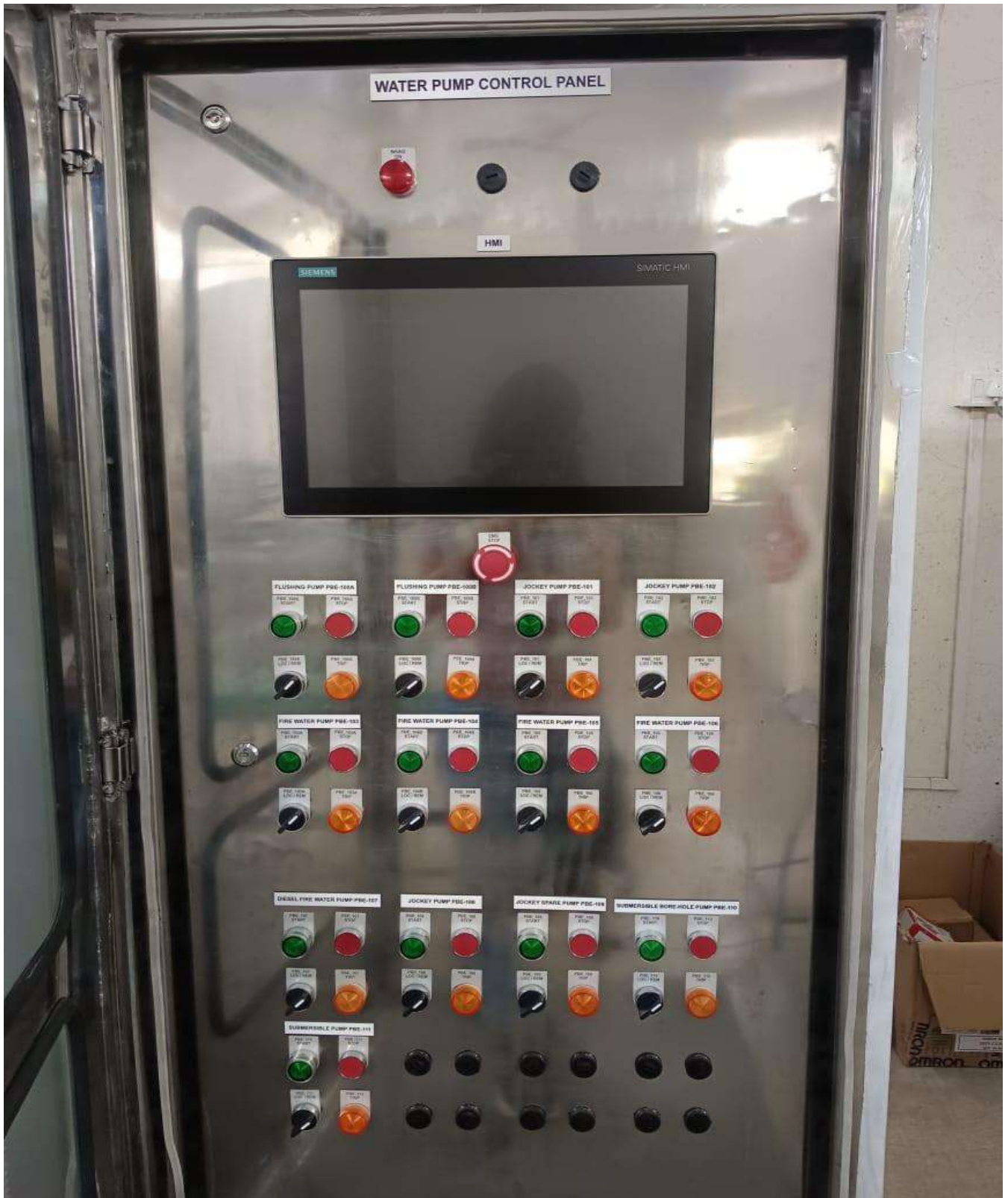
Figure Final water pump Control Panel
