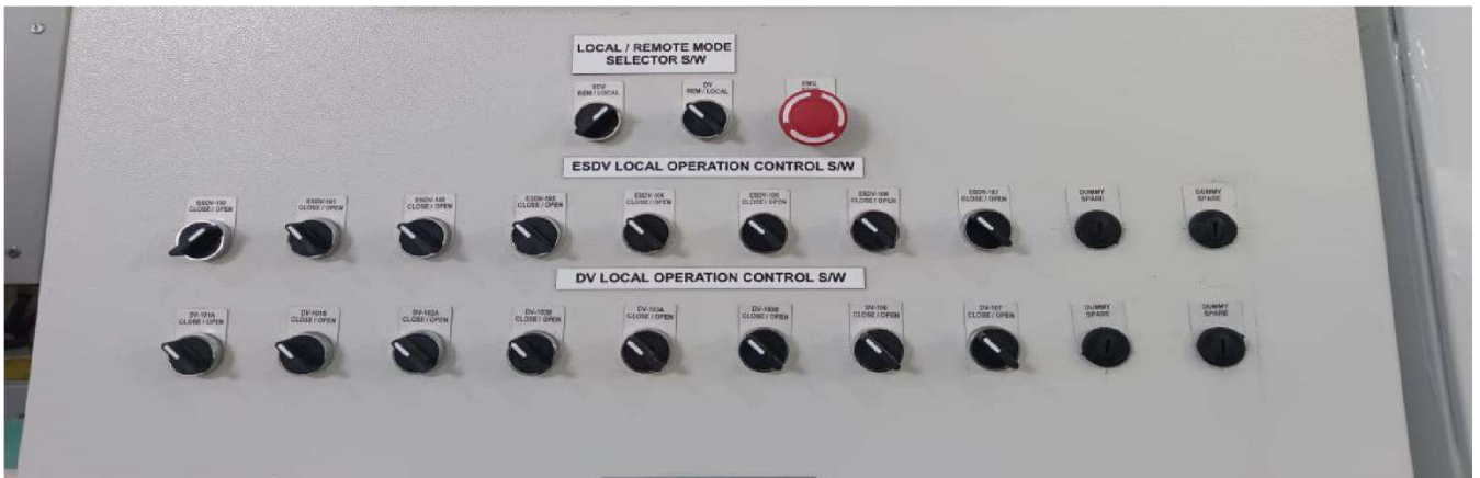
Figure Final Gas and flame Control Panel
