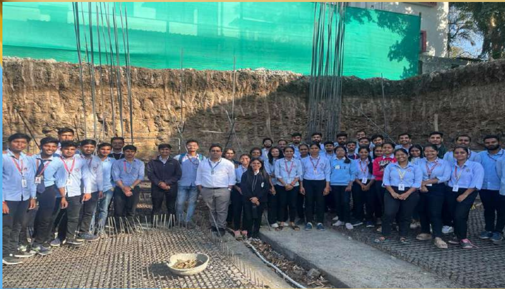
Design of RC structure Footing Visit at Boys hostel MVPS"s KBT COE Nashik Date 22/02/2024
