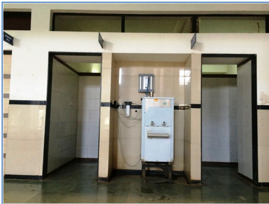
Fig 4.1.7. Water purifiers at each department
