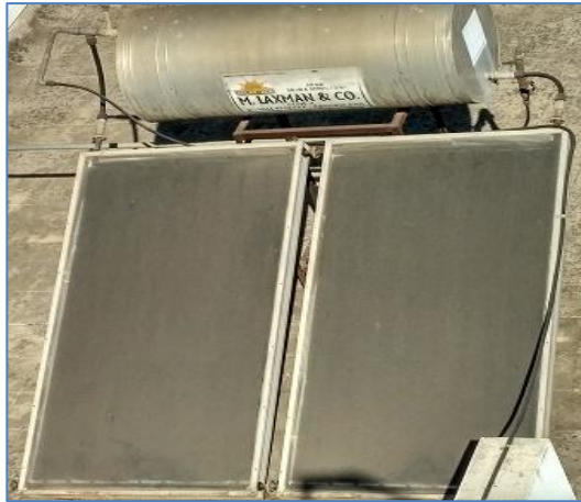
Solar Water Heater:
