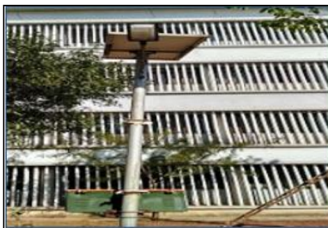
Solar Street Light:
