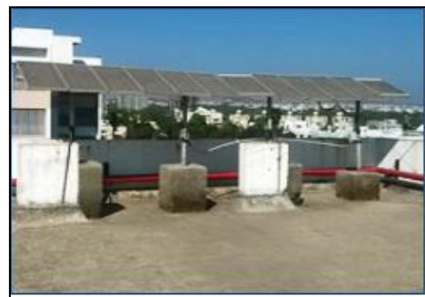
Solar PV Panel:
