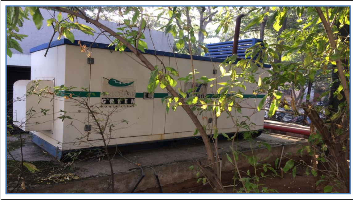
Fig 4.4.4.(B) Generator at safe location
